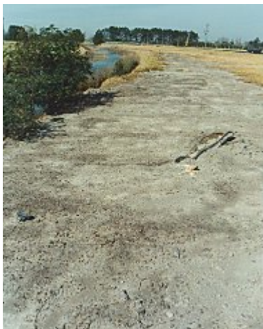
Acid sulfate soil damage at Greenwell Point. Photo: Allan Lugg
