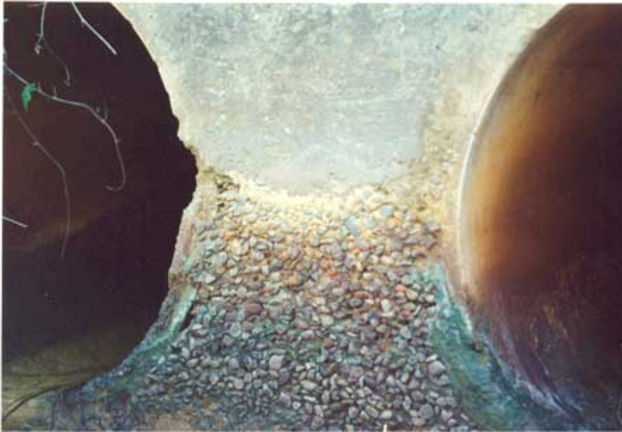
Concrete cancer in pipes Fernbank Creek, Hastings River floodplain, NSW 2001 Photo: G. Atkinson
